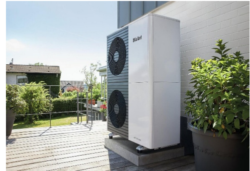
Typical Outdoor Residential Heat Pump Systems Equipment
